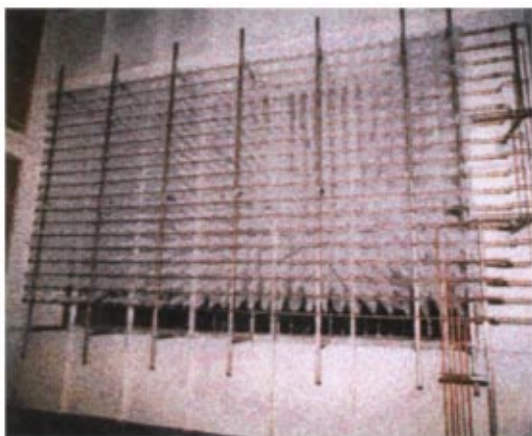
Fig. 2 Fog nozzle manifold operating in the inlet duct of a GE-7EA gas turbine
