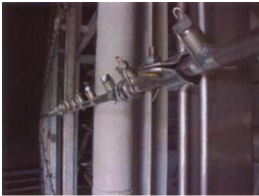
Fig. 12 Lock wire arrangements
