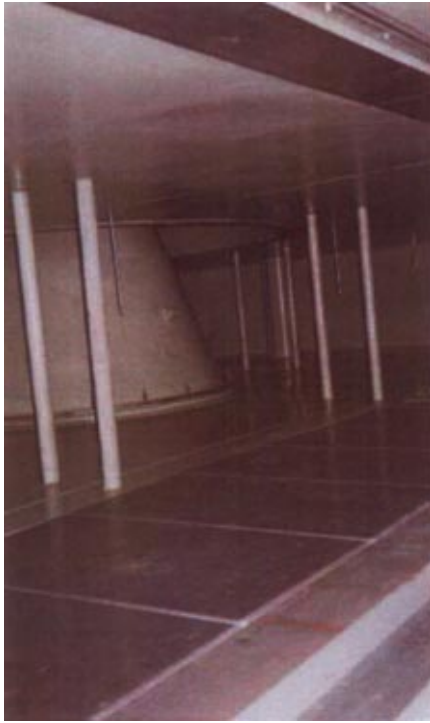
Fig. 14 Duct support structures like those shown here can collect fog and result in excessive pooling of water. Such obstructions must be taken into account when designing the nozzle manifolds.
